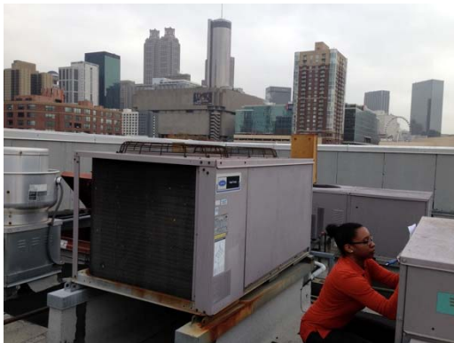
Figure 3: Rooftop HVAC Systems
