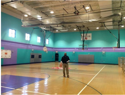
Figure 1: Gymnasium with New LEDs
