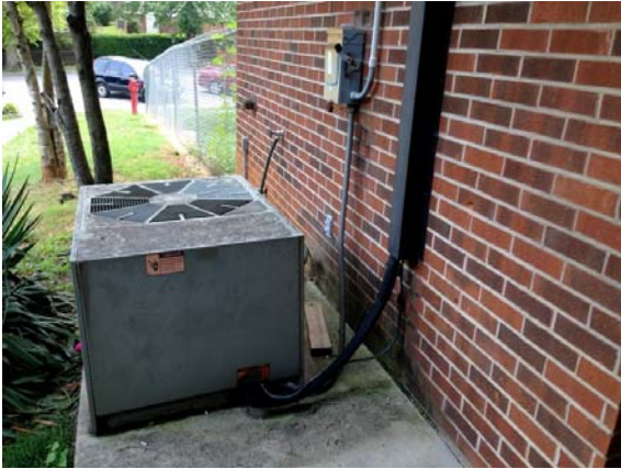
Figure 1: Old HVAC Example
